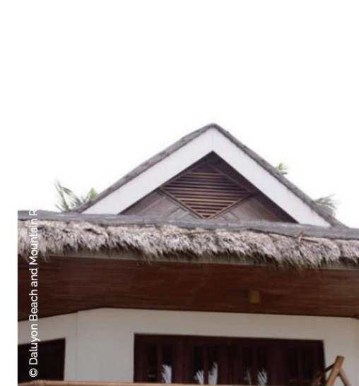
Louver ventilation installed on the roof of a guest room
